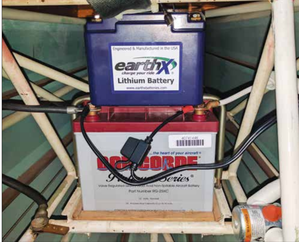
Size matters: The Concorde lead acid battery measures 7.50x4.57x6.81 inches and weighs 23.5 pounds. It was replaced by an EarthX ETX680C, which measures 5.9x3.4x4.5 inches and weighs 3.9 pounds, a weight savings of 19.6 pounds.
